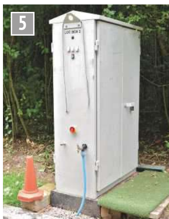
At the extremity of the track from the station this new water, air and power box allows drivers to stop and recover without holding up any following traffic.
