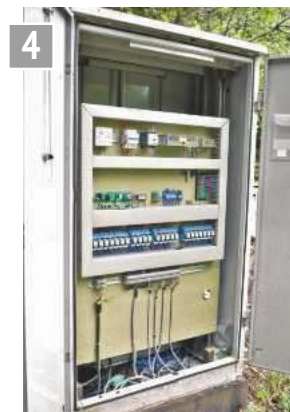
One of the excellent control boxes built for the new track.
