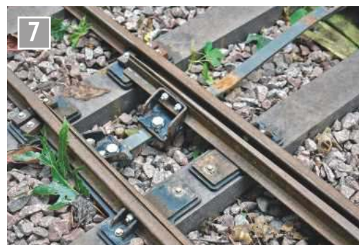
The substantial connectors on the moving blades of the points.
