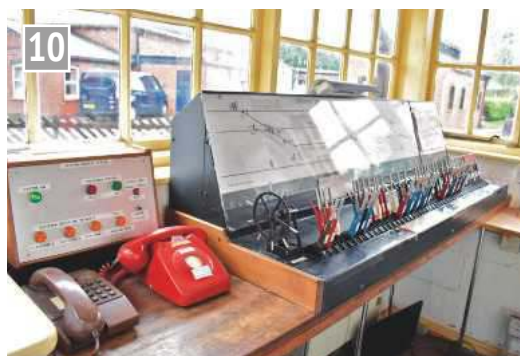
The signal box lever frame and controls including the super little crossing gate control wheel.
