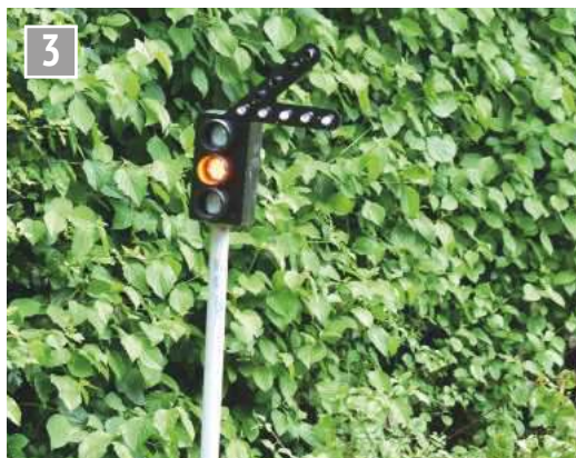
One of the new colour light signals built and installed by the club for the new extension.
