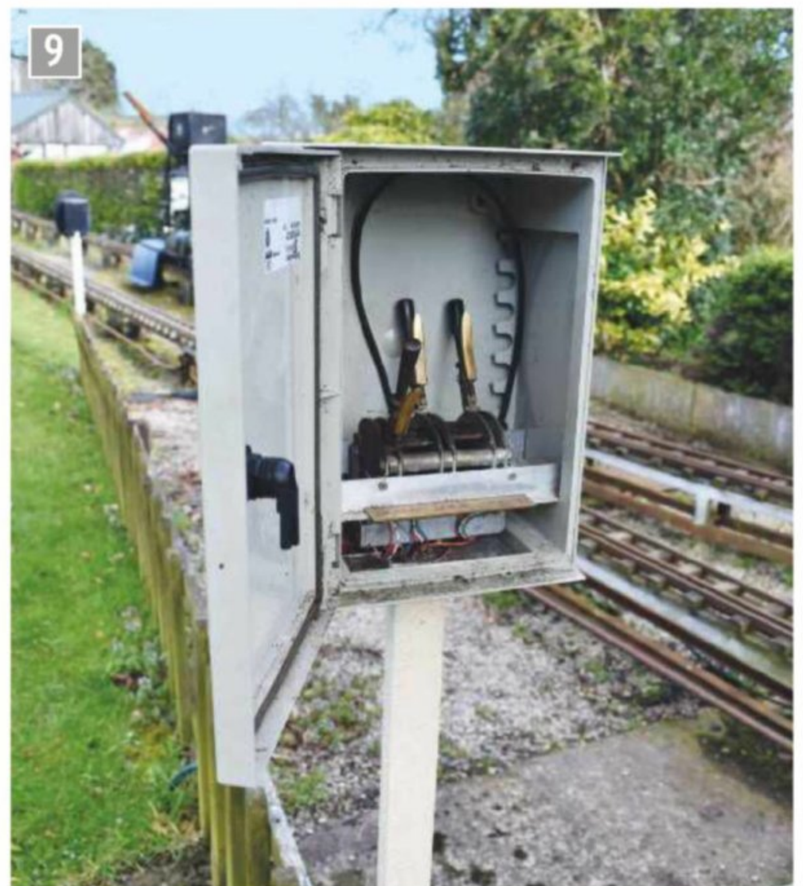
Traverser control box.
