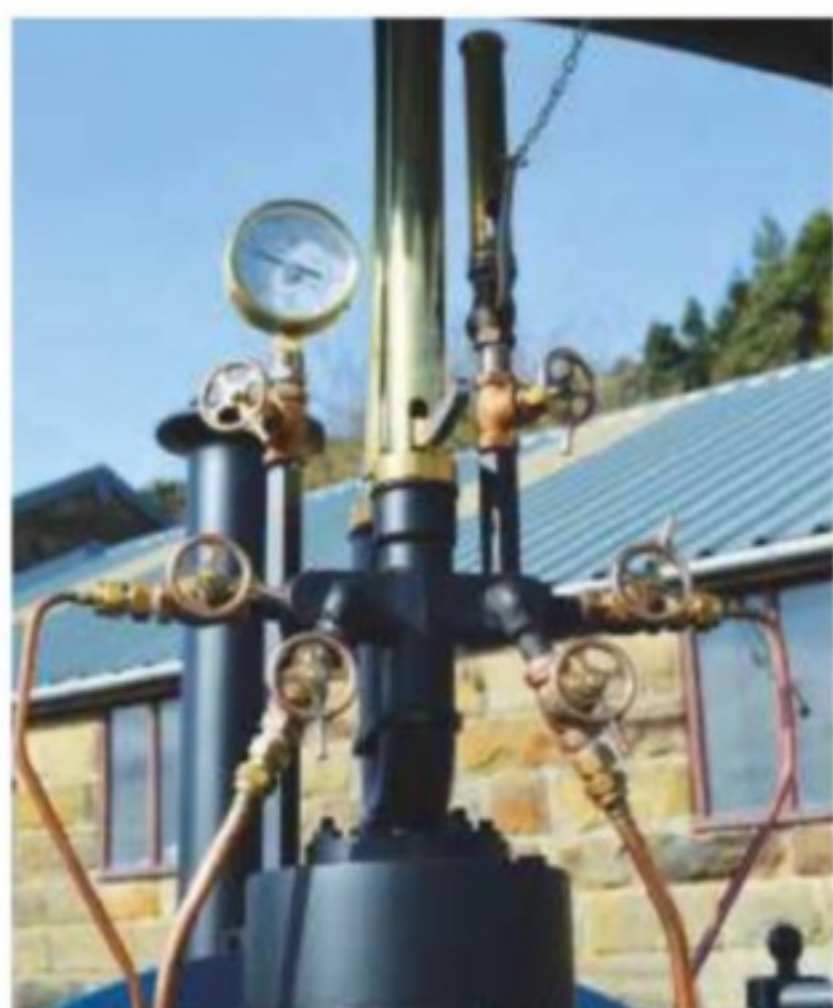
The steam manifold is shown in this view, attached to the rear column of the safety valve casting. The lower pair of take-offs are for the injector steam feeds, whereas uppermost we have (L to R) the blower; the whistle and the steam draincock feed (the latter certainly a non-original feature).
