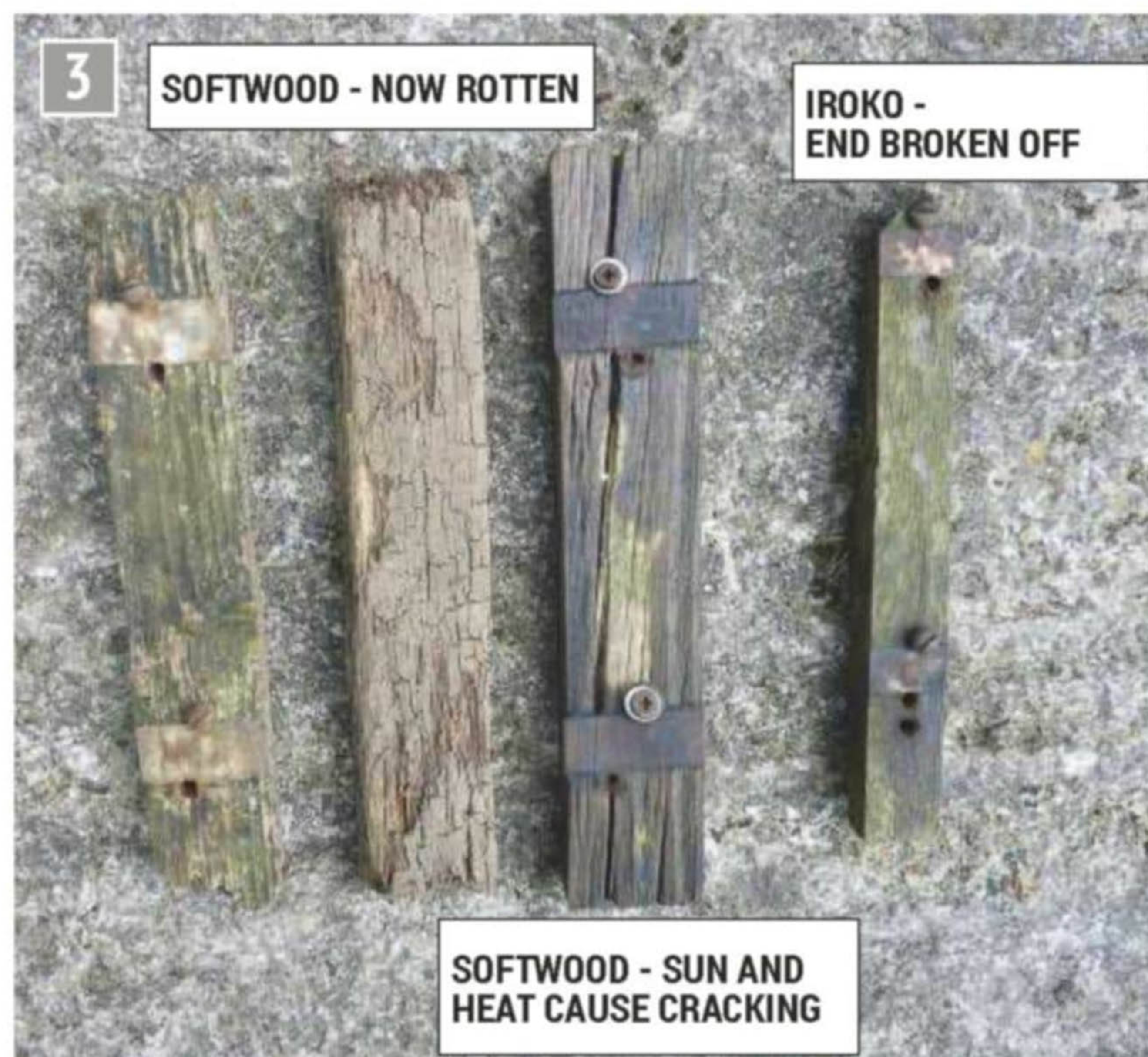
More rotten sleepers.
