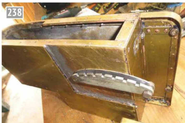
238 Cut-out in driver's side tank.
