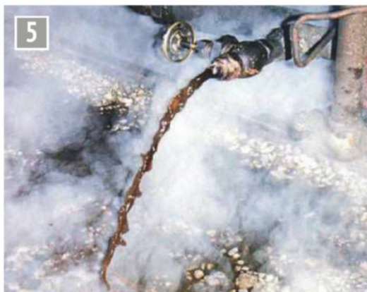
Even darker brown is acceptable! This image of just-off-of-steam hot boiler water draining shows the sludge and colour associated with the treatment.
