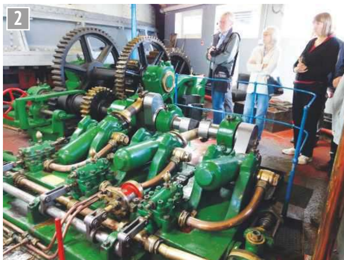
Swing bridge hydraulic machinery. (Photo courtesy of Malcolm Phillips.)
