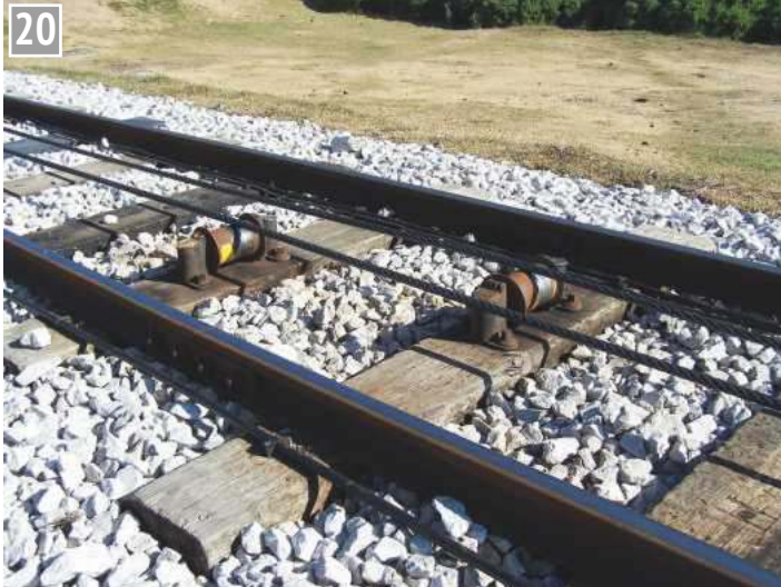
Horizontal rollers guiding the cables on the straight sections.
