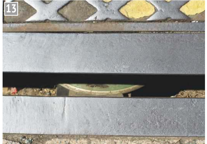
One of the guiding sheaves in the conduit.
