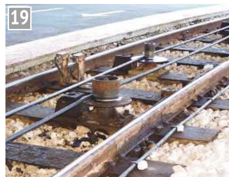
The flanged pulleys guiding the cables on the curve.
