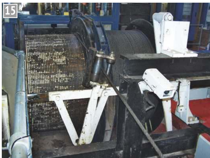
The guide rollers on the Upper Section winding drums.
