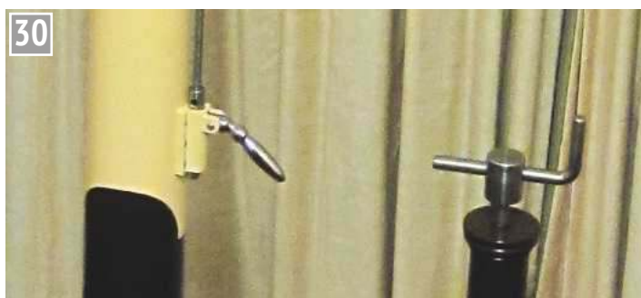
Lock and water control handles.
