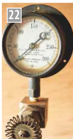
Pressure gauge from a Parsons turbine in Lots Road power station, installed about 1930 (photo by Duncan Andison, Izel Photography).
