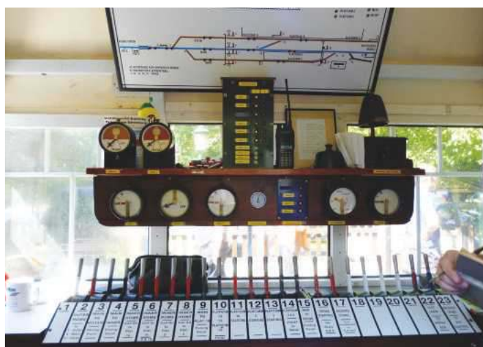
The railway is fully signalled and has three operating signal boxes, along with some automatic systems. Here is the interior of Harvesters Station Box.
