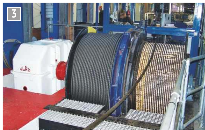
The lower section winding drums.
