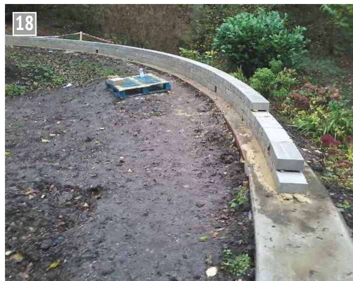
The gaps at the base of the wall for the wildlife.
