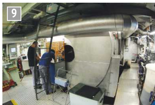
The oil fired boiler.
