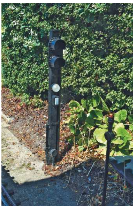
Part of the control system for the track traverser system.
