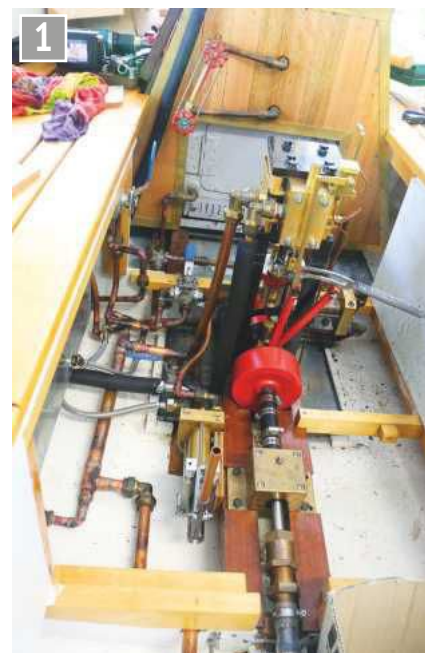
Plumbing in Brahminy.
