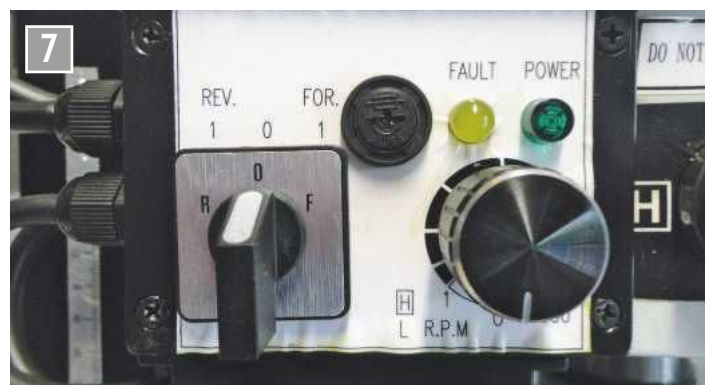
The control decal was slightly damaged by the rust preventative oil.
