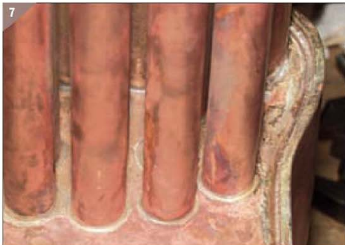
8. Tubeplate not square to the wrapper!
