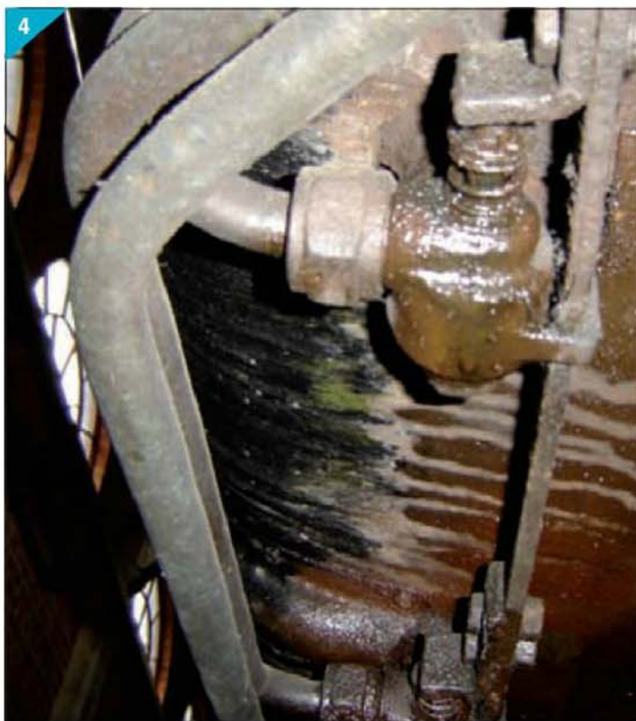
3. The underside of the rear draincock. 4. The underside of the front draincock.
