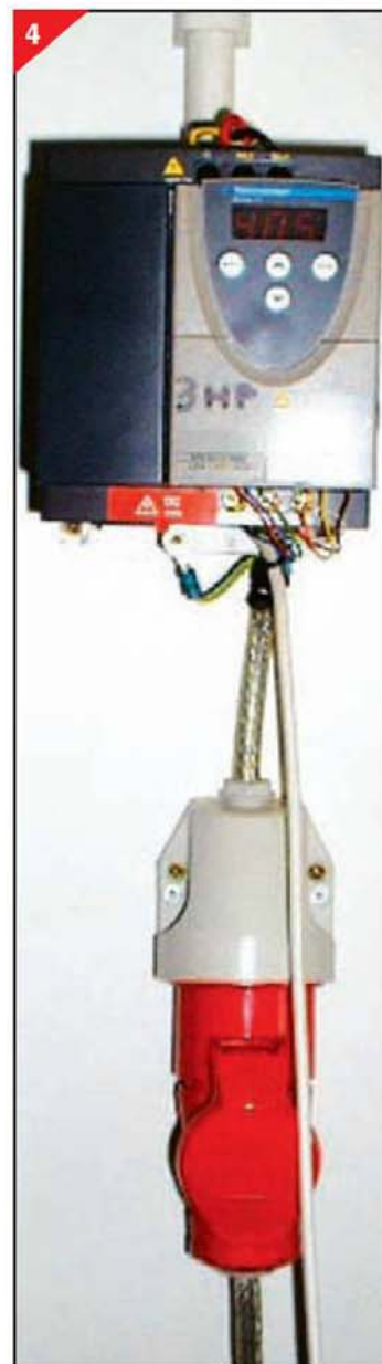
3. Remote control box for operating inverter from the machine.
