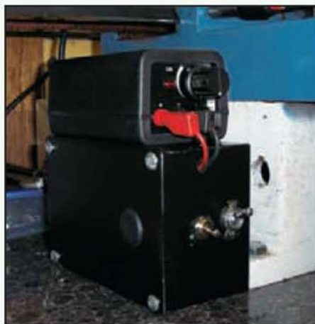
The electrical control system for the installation rests near the machine.
