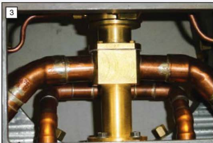
3 The smokebox front view with the strongback removed to show the pipework.
