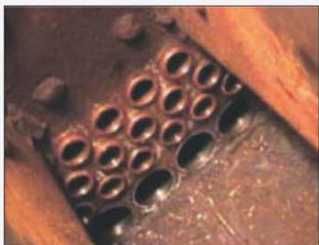
Fortunately the old tubes were removed without damage to the tube plates.
