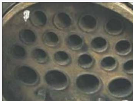
Seventeen years of heat and corrosion!
