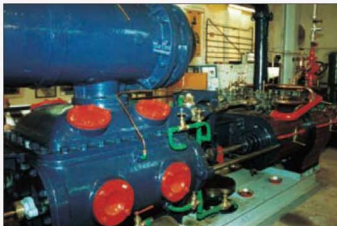
Horizontal Triple Expansion Duplex Pumping Engine built by J. Simpson of Pimlico in 1889. It is reputed to be the first triple expansion engine built by this company. The cylinder seen above the twin rams is the condenser.
