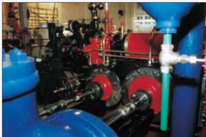
Another Worthington-Simpson engine on display is this Horizontal Compound Engine of 1918 as supplied to Denge Pumping Station.
