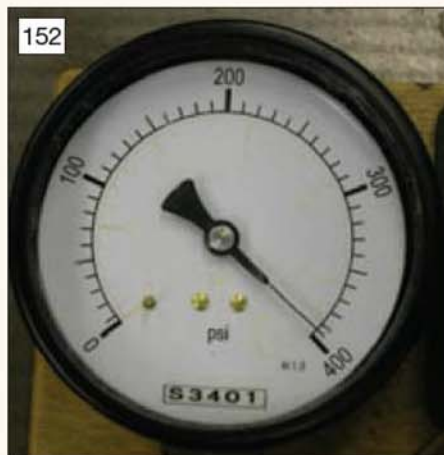
Pressure gauge recording 400psi with no sign of distress from the boiler.
