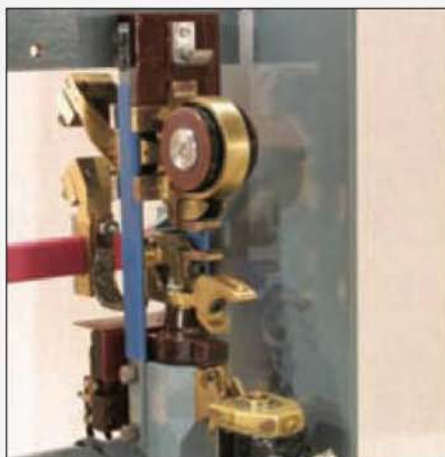
General view of the contactor with the test blow out coil fitted.
