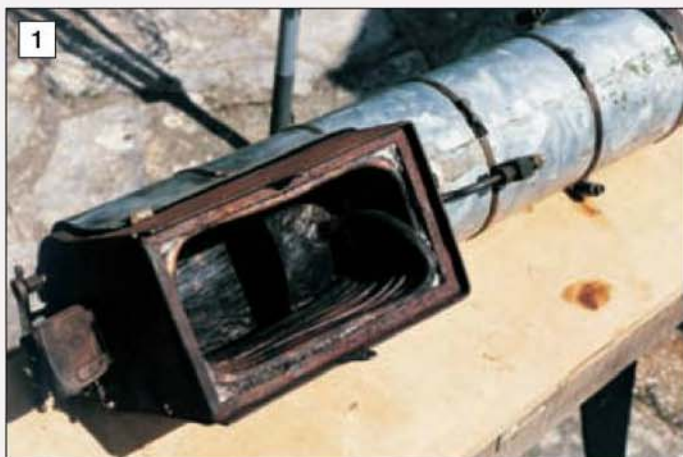
Normal fire tube boiler, but with...
