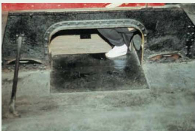
Shovelling plate and coal space.
