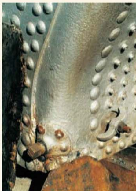
Close up photo of the front right hand side of one of the boilers near to the foundation ring.
