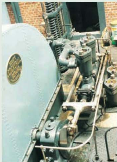
The Pelton wheel and hydraulic pump used to make up for any leakage in the hydraulic system.
