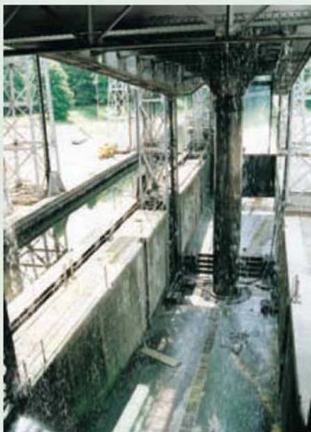
A view underneath the trough at the top lift, showing that the seals between the trough and the canal do leak a little.
