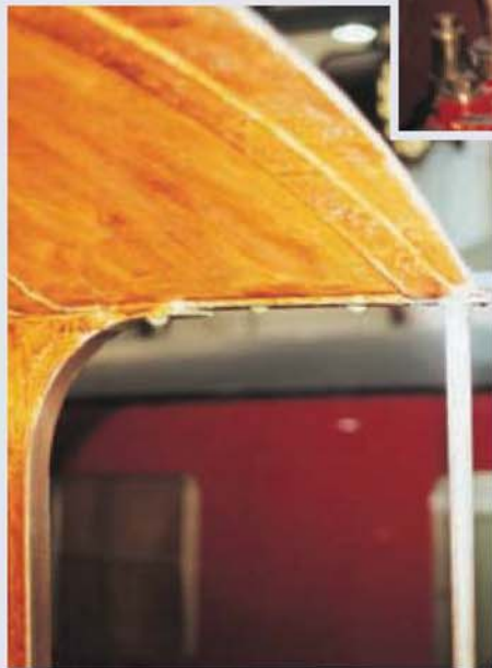
Inside the cab of No. 103; note the bracing doubler inside the rear edge of the roof.
