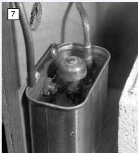
A Spam can makes a fine hot well. The snifting valve is mounted above the water level so that water discharge can be observed.
