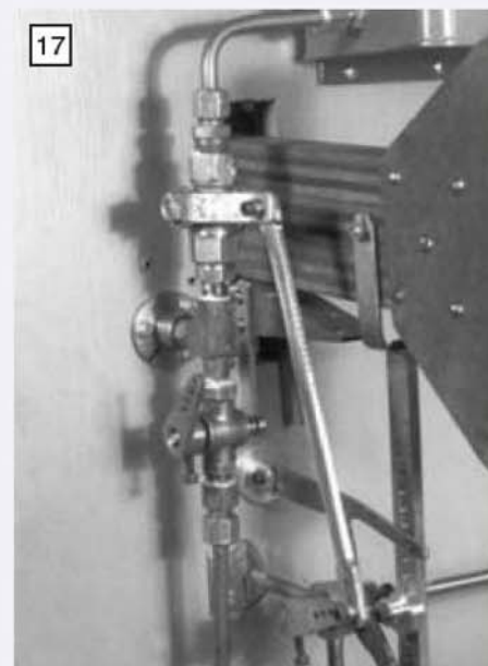
17 The injection water valve must be free working. The lower valve keeps the boiler from overflowing when the beam is up.
