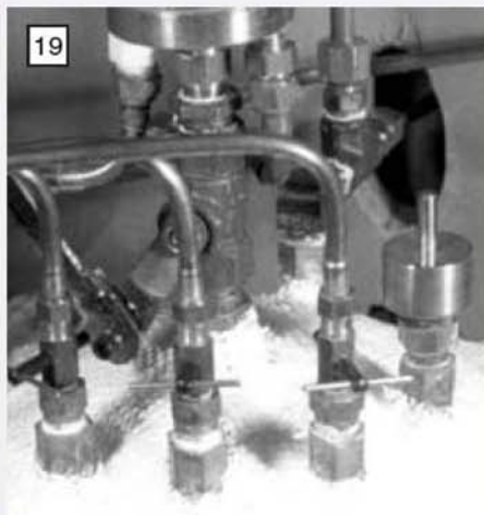
19 The boiler top gets crowded. Pressure in the boiler can be adjusted by substituting weights on the safety valve.
