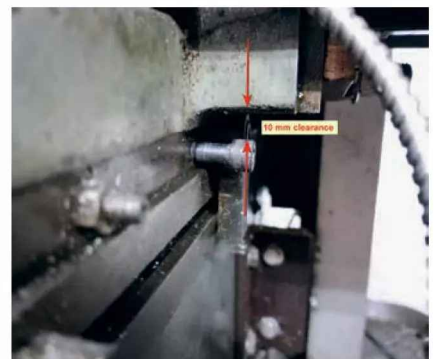
Photo 2: Limited clearance limits the obvious solutions.
