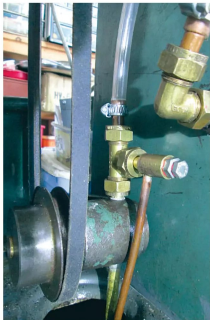
Photo 16: Suds pump remounted showing relief valve and return pipe.
