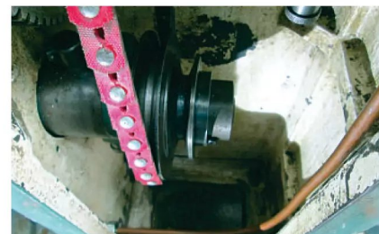
Photo 19: Copper pipe routing in the man column.
