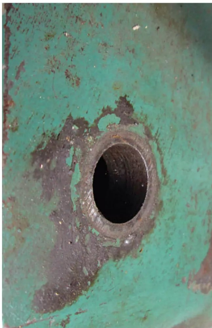
Photo 17: Large hole in the top of the mill main casting.
