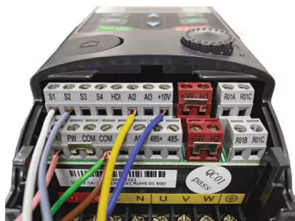
Photo 2: Remote/Inverter Terminal Connections.
