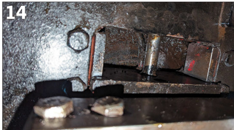
PHOTO 13: The final, butchered tooling that was required to tighten the bolt.
