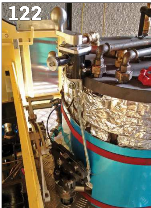
PHOTO 122: View of whole regulator assembly on the boiler.
