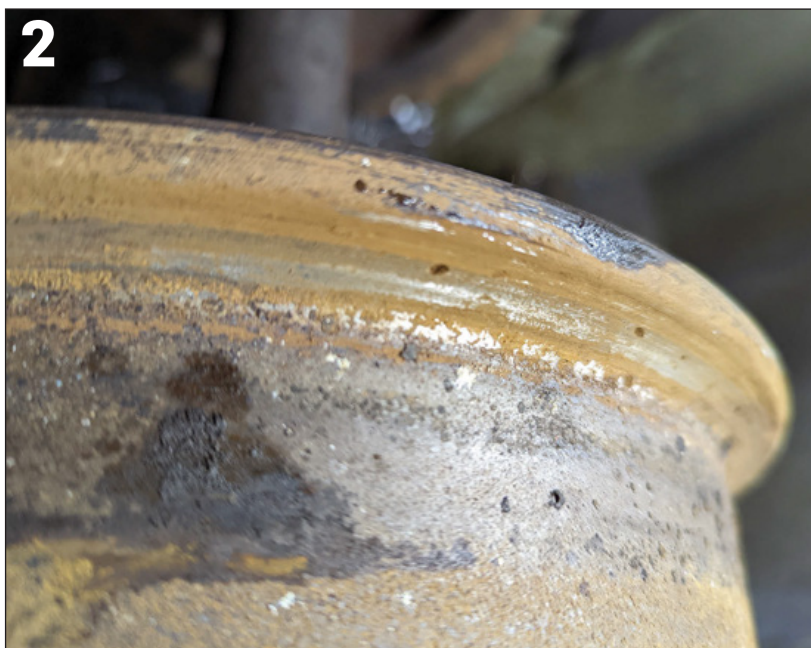
PHOTO 1: A carriage wheel with a welded-up root radius, note the strange wear patterns visible.
