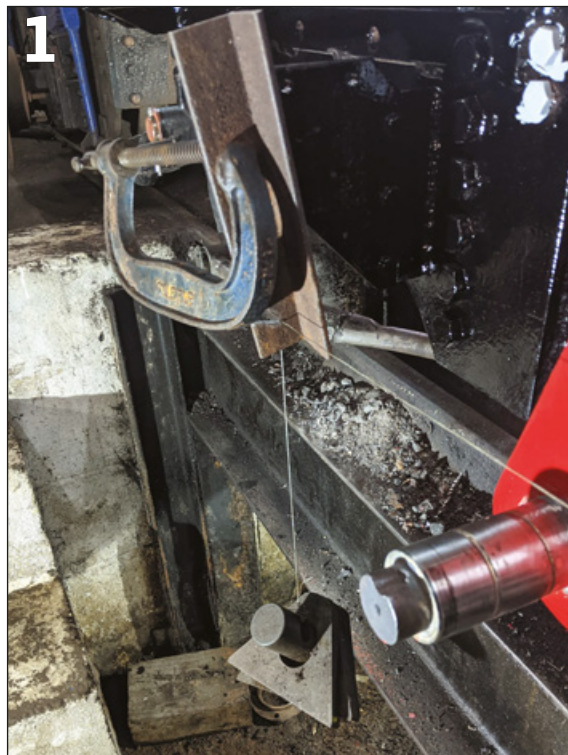
PHOTO 1: Cylinder lining rear bracket, showing V-notch and clamp holding it in place on framework. Note also the tensioning weight.
