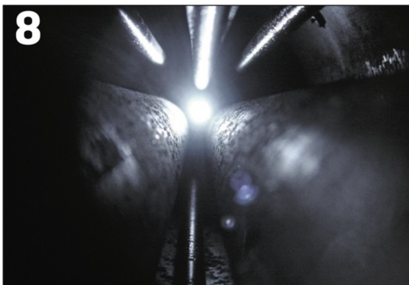
PHOTO 9: Rusting joints in turnouts do need little oiling now and then...
