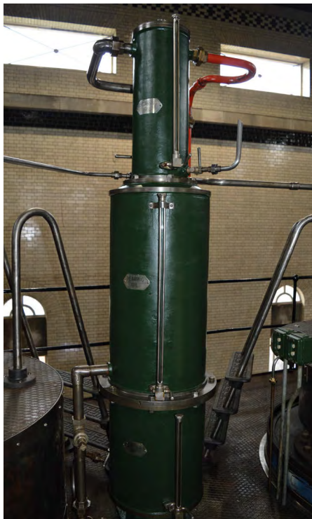
ABOVE – The oil reservoir tower for Engine No. 7 is shown in this view. The upper two reservoirs were filled with low viscosity bearing oil (feeding the gravity lubrication system), whereas the lower reservoir was filled with high viscosity cylinder, or 'steam' oil, feeding the mechanical lubrication system.
