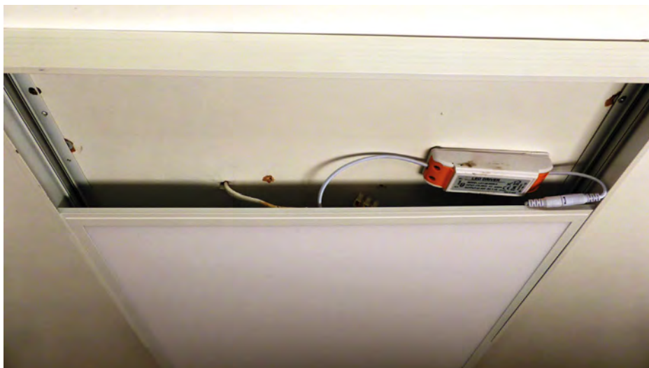
ABOVE – PHOTOGRAPH 14 600x600mm LED light panel.
