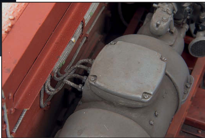
The cables on the wall were connected up to the outlets on the back of the generator
