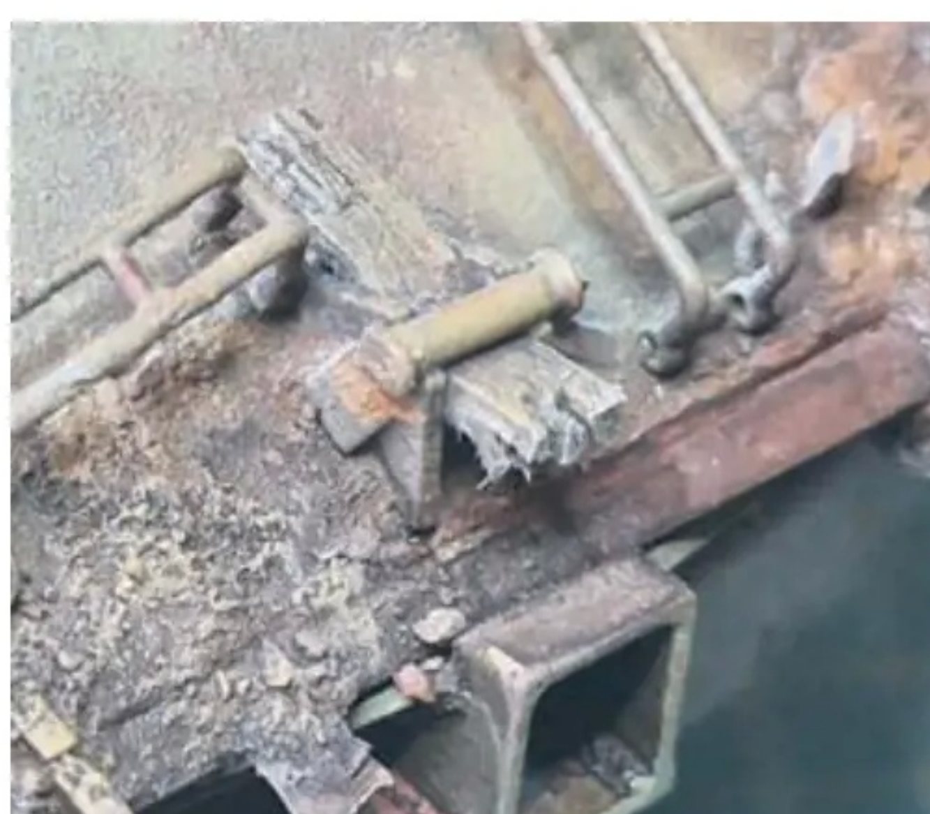
wooden plank jammed into the front brace.
