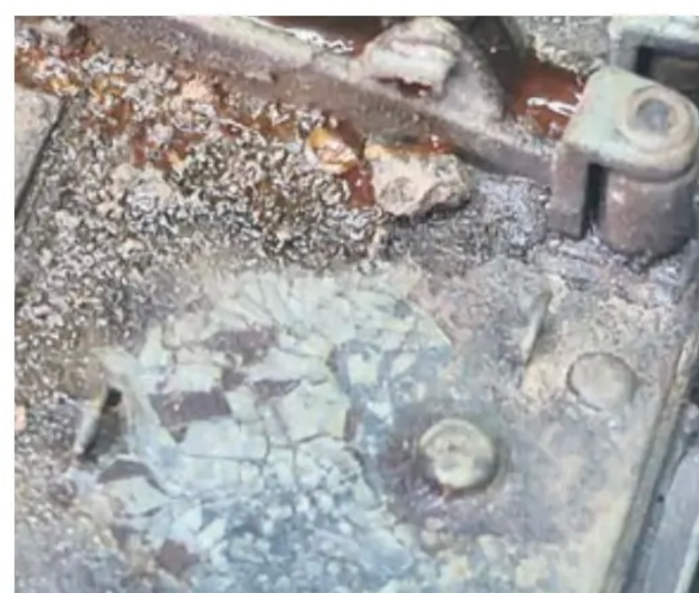
Mud, stones and chipped paint on the hull top.
