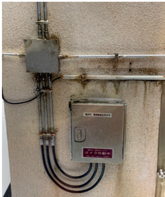
▲ Cables and wires by Tokyo Build
