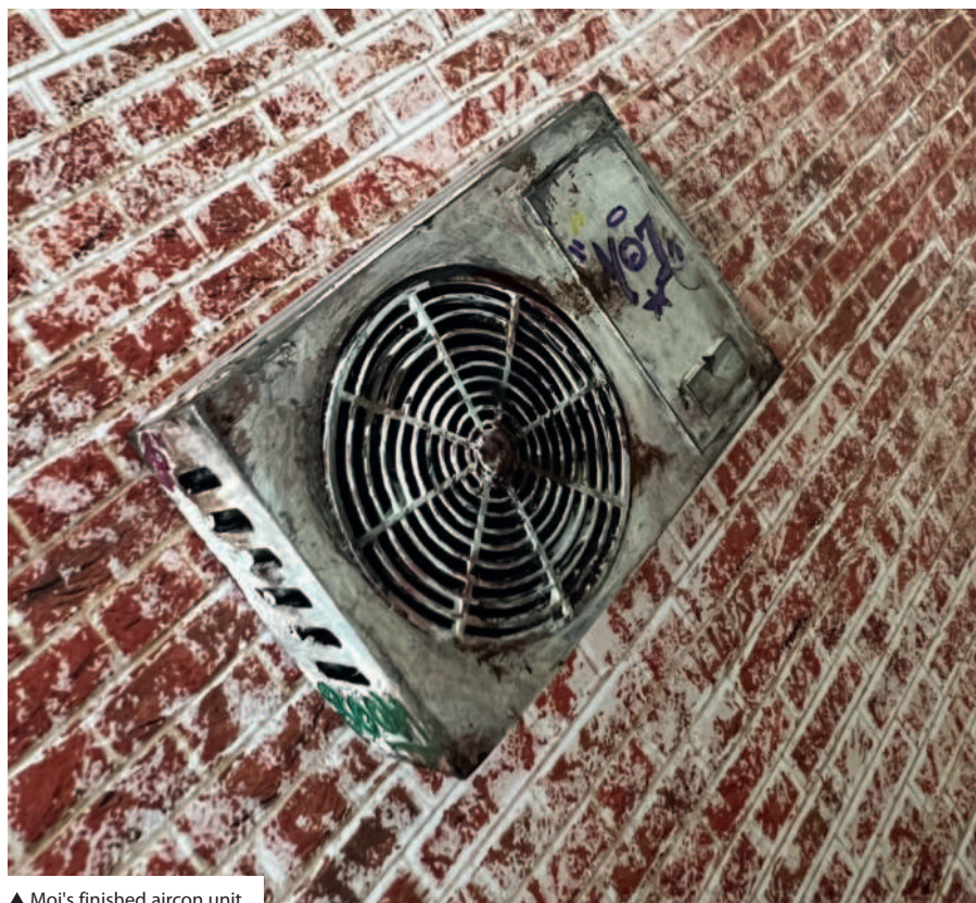
▲ Moi's finished aircon unit
