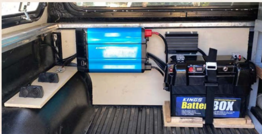
For extended periods out bush: a deep cycle battery, solar charging and inverter.
