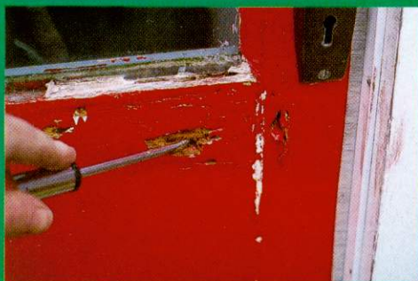
Initially the decay appeared minor
