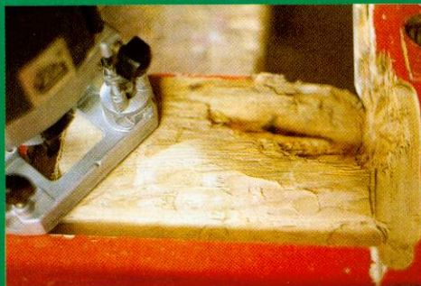
Decay cut away to reveal sound timber
