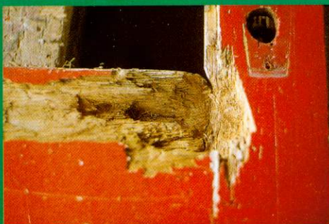
The stile was also decayed
