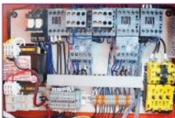
Clear-cut DC control cabinet
