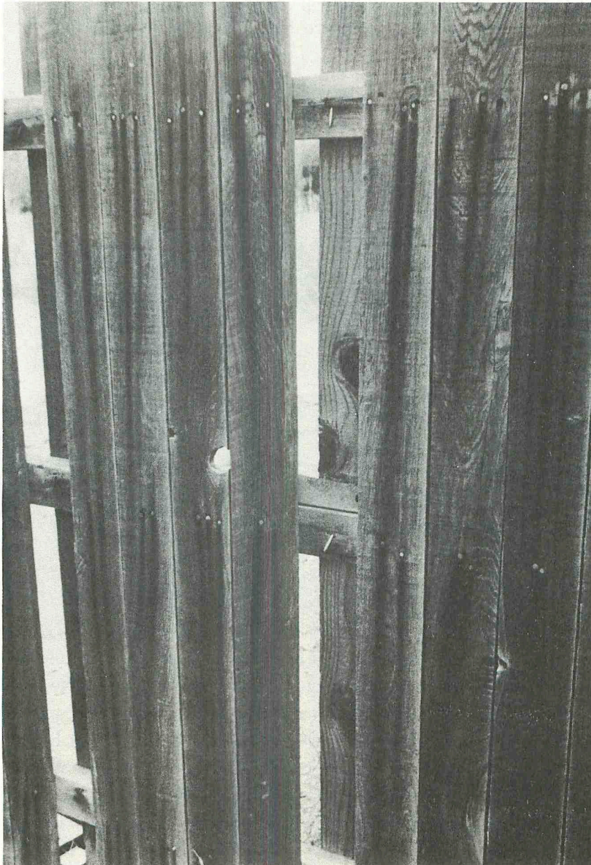
Illus. 27. In this vertical-board fence with panels that alternate sides, you can see the clinched nails on the rails, as well as rust streaks from the mild steel, uncoated nails.
