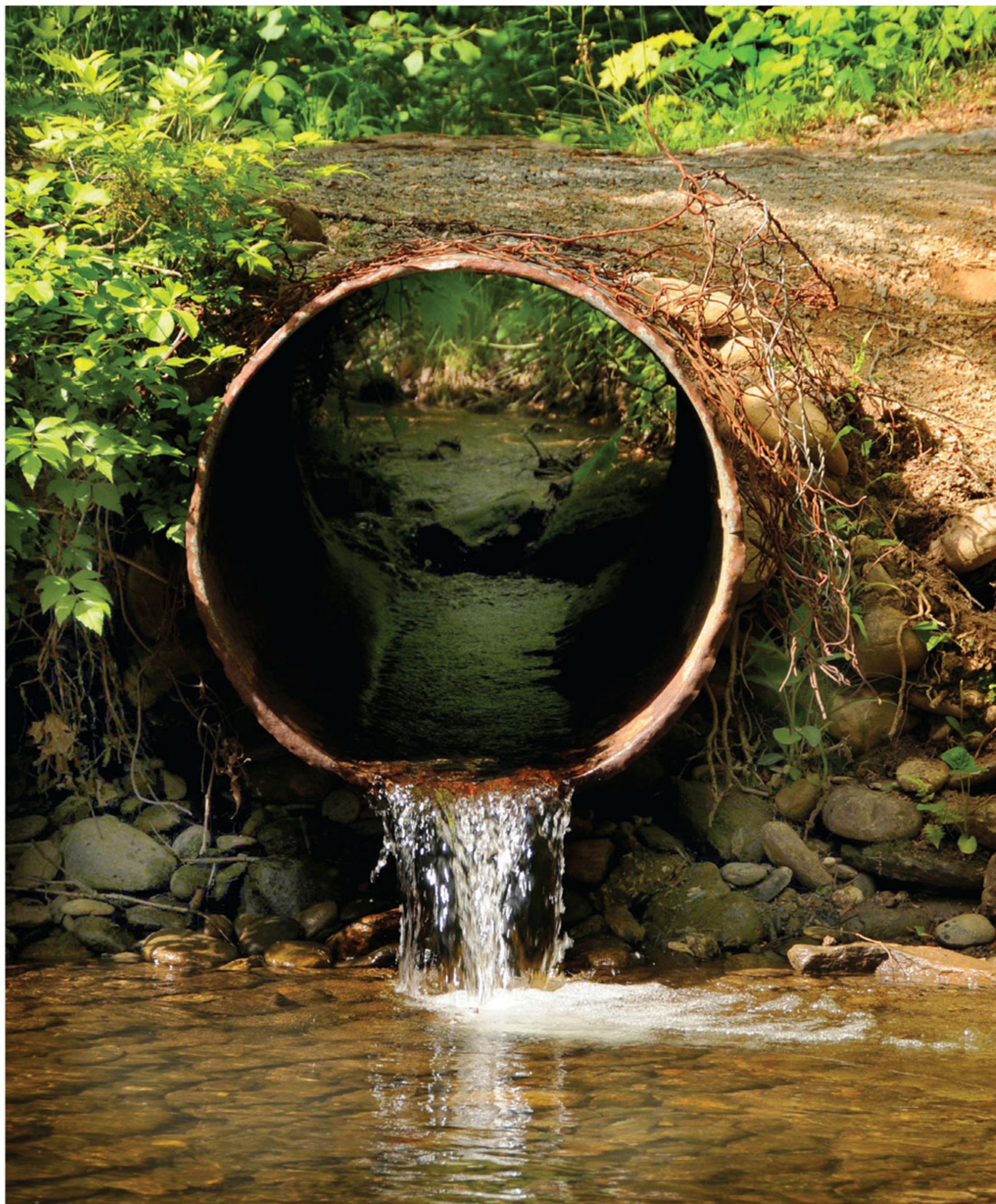
It may be time to replace the stones surrounding this water drainage pipe in North Carolina.
