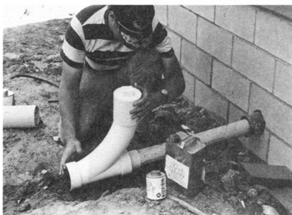
All drain pipes, including the house sewer, need clean-outs. This one is made from a 4-inch, long-sweep PVC sewer Y adapted to the 3-inch house drainage system 5 feet beyond the foundation. (Photo by Genova, Inc.)
