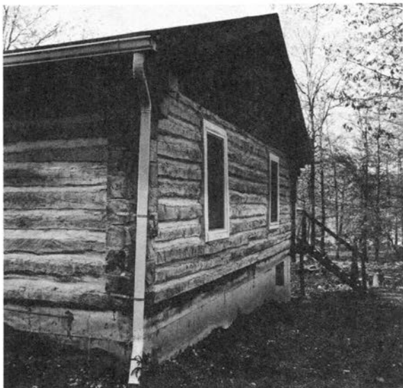
A proper roof drainage system can protect the soil surrounding the house from erosion and keep water from splashing up on logs.
