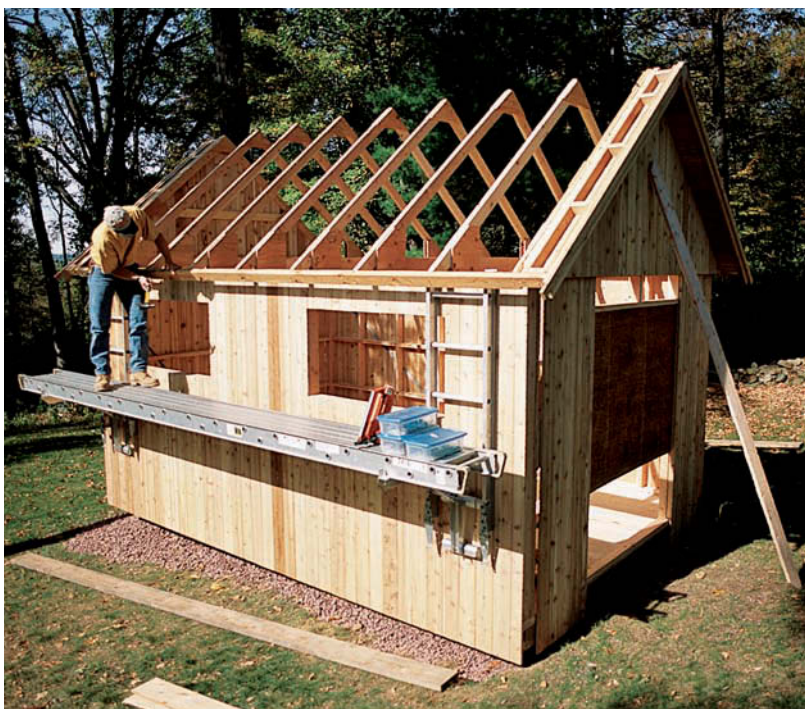
The gable roof of this shed was framed with site-built roof trusses; note that there's no ridge board running along the peak.
