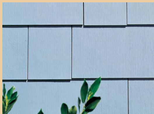
What appear to be individual wood shingles installed with staggered butt edges are actually 4-ft.-long fiber-cement planks.
